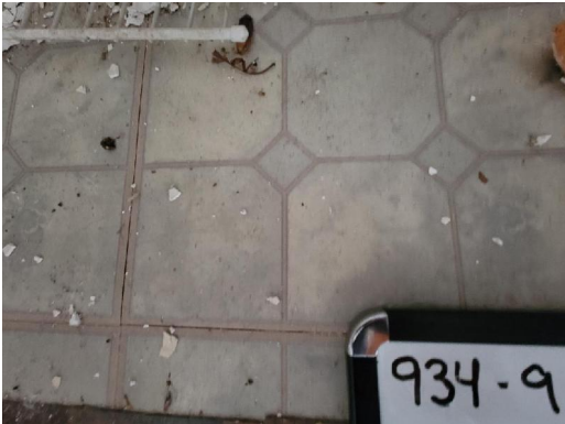
934-9 12"x12" Floor Tile/Adhesive Interior Bathroom (Top Layer)
